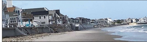
Ongoing efforts are underway to repair and replace aging and damaged seawalls in front of beachfront homes. A portion of the wall has been repaired, and officials plan to stabilize the beach in front of the wall.
